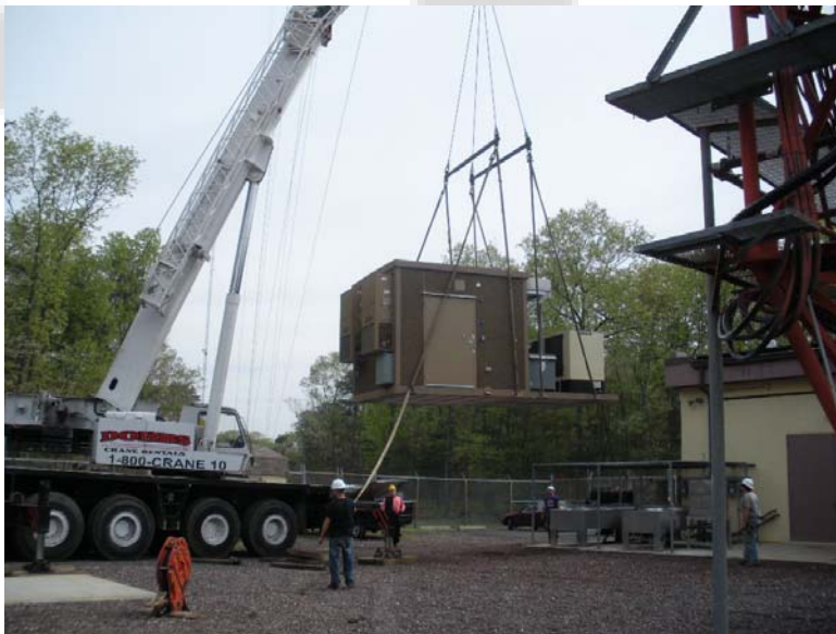
Installation of a FLO TV compact shelter. This shelter is fully integrated on a prefabricated reinforced concrete pad with the heat exchanger, transformer and generator already installed and wired ready for testing and commissioning.
