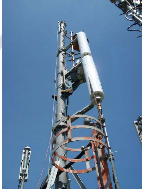
Installation of a UHF antenna on a custom KMB designed tower extension mast.
