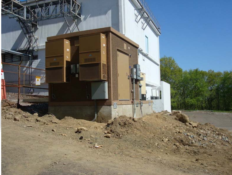
FLO TV shelter on a reinforced concrete foundation with integrated back-up generator.
